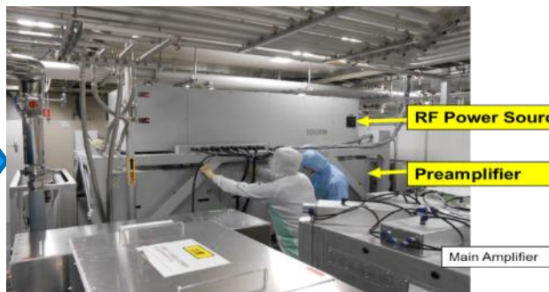
1st Amplifier installation in 2015
